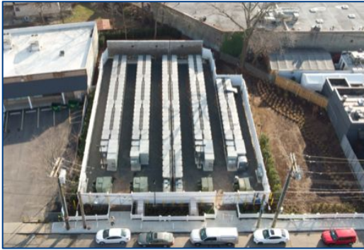
The 1st and largest community-scale low-carbon electricity generation project (Staten Island)
