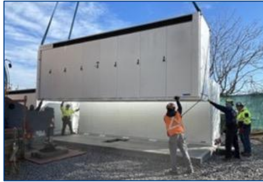
The 1st Tesla Megapack, community-scale battery storage project (Bronx)
