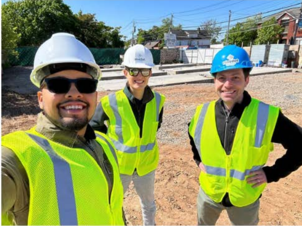
NineDot team members at one of our Staten Island projects, ready for battery placement.
